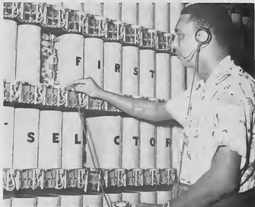
MAKING A routine test on selectors is C. HACIENDO UN test di rutina ariba selector Pierre of the telephone exchange. These selectors are part of the equipment that provides automatic service.
